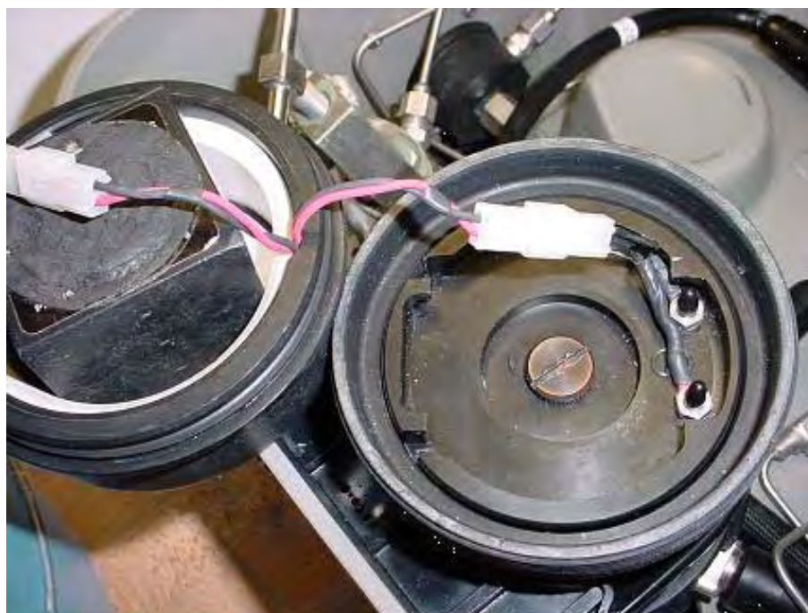
Figure 21. Improperly spliced connectors in an electronics pod.
